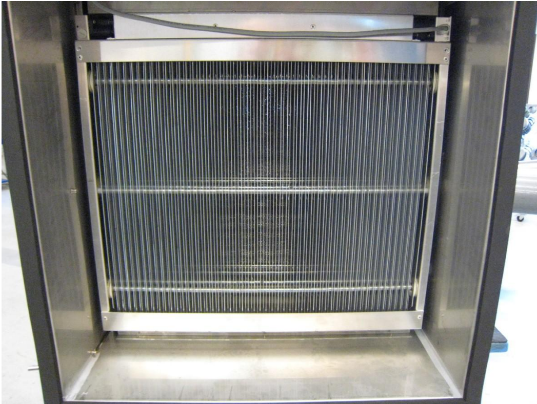
Fig 7. Three FE600 mounted in series in the duct section, back side
